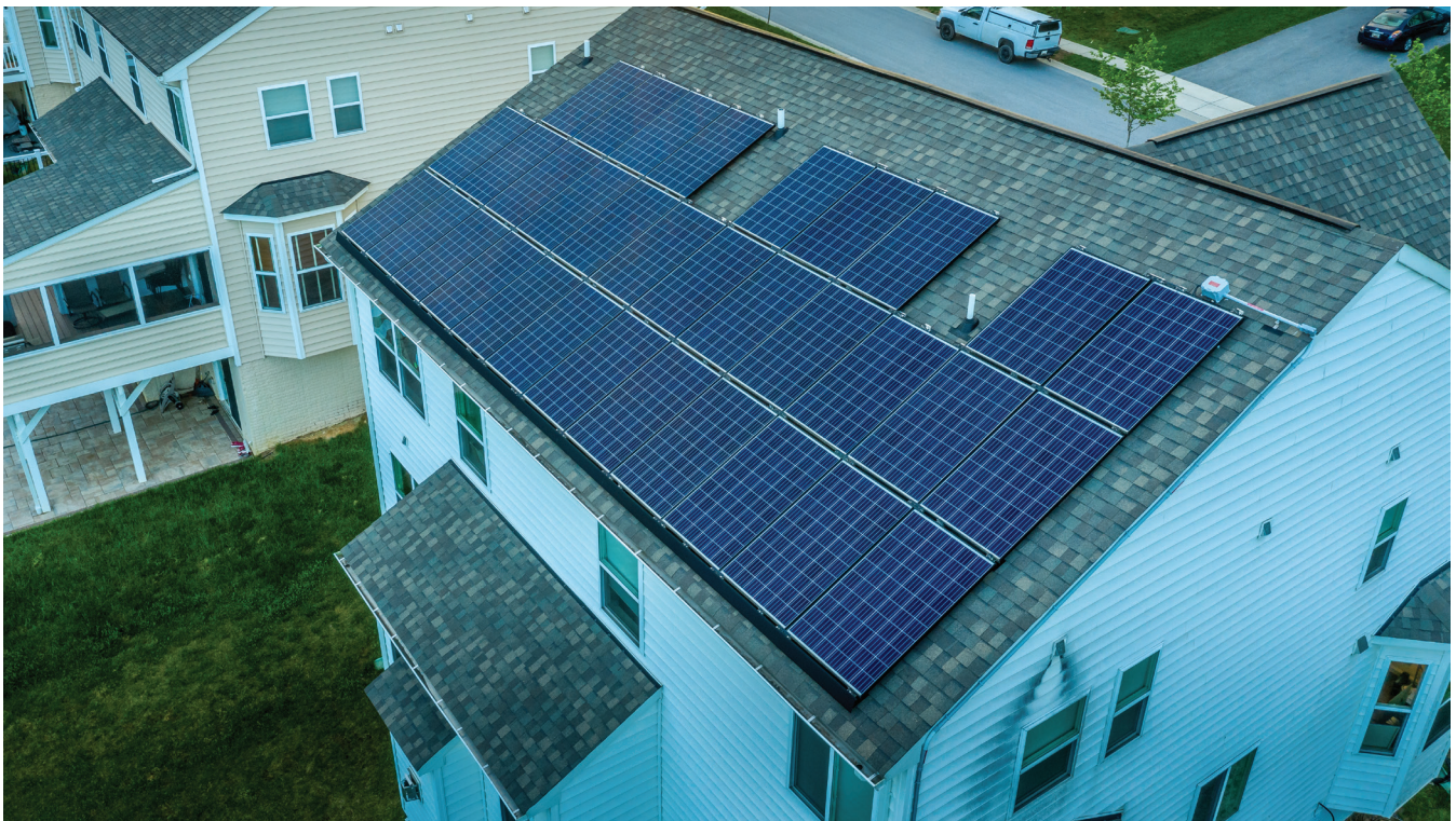
Solar panels on the roof of a home in a subdivision in Maryland. This image is used under license from Shutterstock.com.
